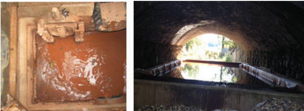
Figure 9: Outfall chamber and clarification tank respectively.
