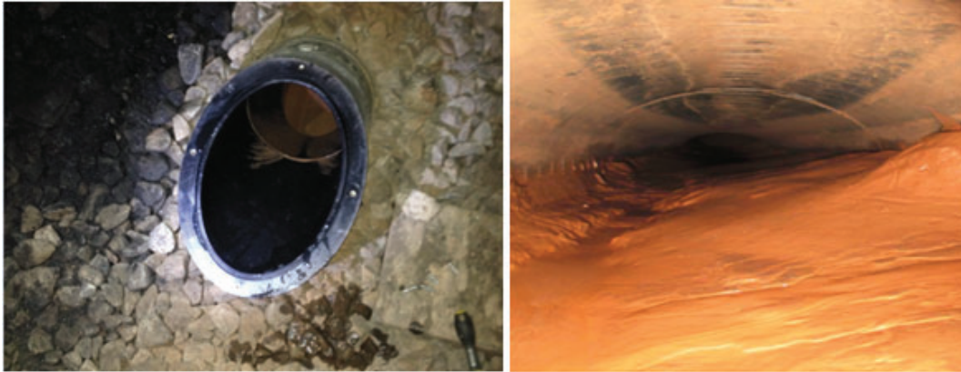
Figure 8: Rodding points in the Up cess showed extensive siltation within the system
