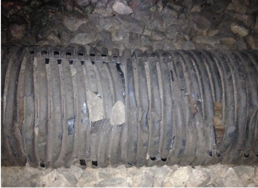
Figure 6: Indicative of high installation and resulting damage to drainage pipes
