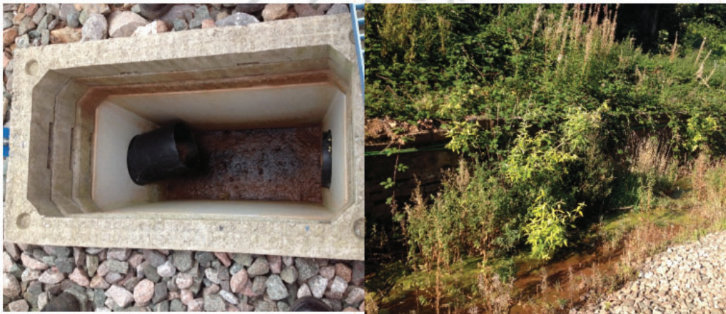
Figure 10: a) Final catchpit (condition indicative of all d/s catchpits) b) standing water observed within the cess
