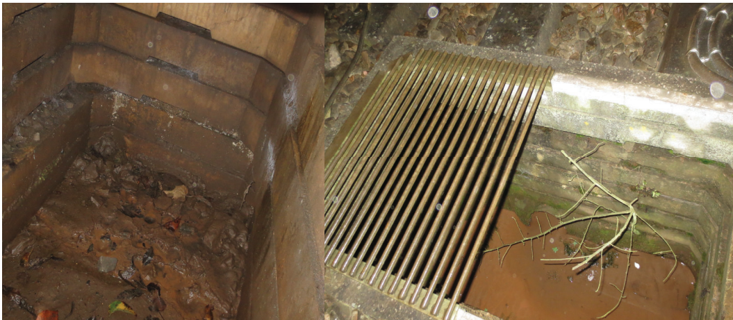
Figure 1: Indicative CAT1.1 catchpit condition
