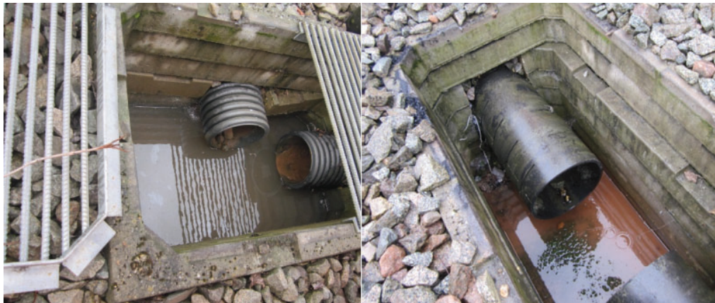
Figure 2: Indicative CAT1 catchpit condition
