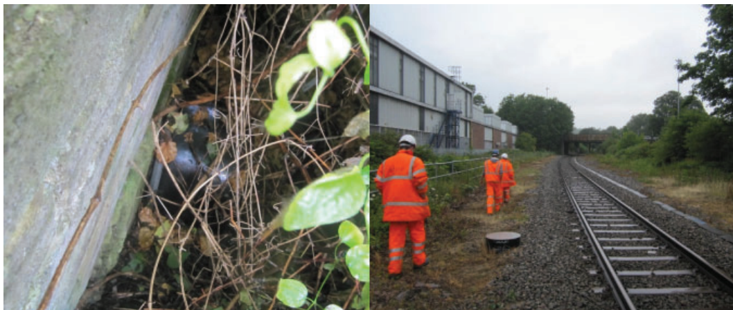
Figure 4: a) Outfall to concrete lined ditch, b) Route showing AQUA SE catchpits in the Dn cess (handrail to LHS of picture is on top of the outfall ditch). Note the lids have now been changed for grated steel lids.
